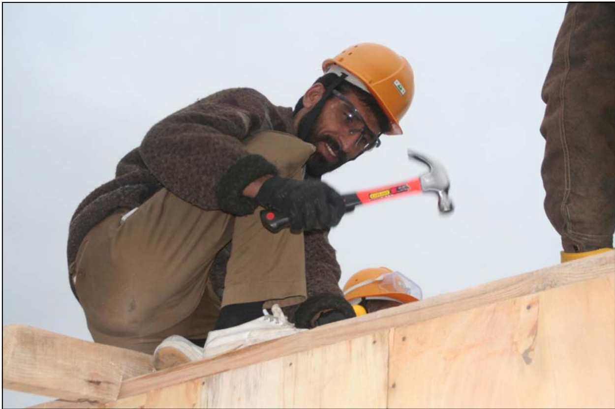
At a skilled labor workshop in Jalalabad, Afghanistan, an Afghan student hammers the roof of a tool shed. The tool shed is one of two hands-on projects conducted at the workshop instructed by Task Force Rugged Soldiers, 36th Engineer Brigade and the 864th Engineer Battalion. The skill labor workshop is funded by the Commander's Emergency Response Program to develop construction skills among Afghan residents.
