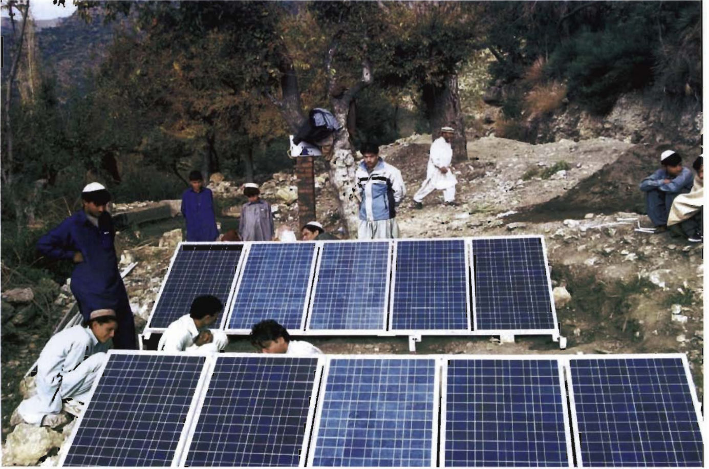
PV Panels at Toda Cheena
