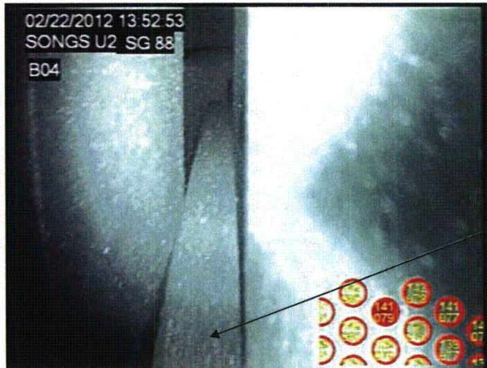
Photo-3 Visual Inspection Image of Outermost Tube Region [Unit-2B]
