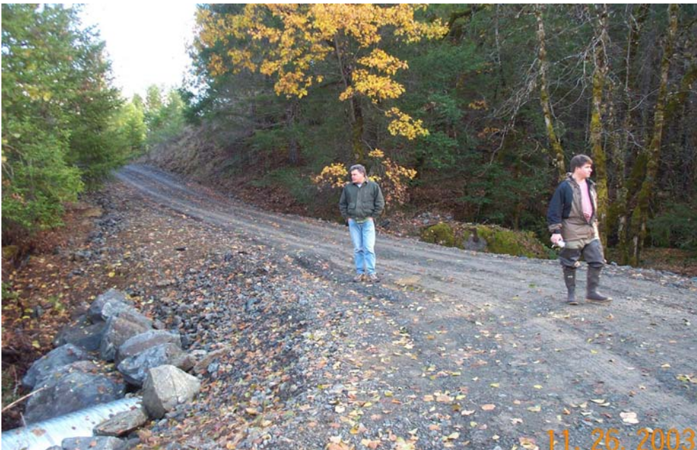
Figure 7. Same tributary as above with 2002 culvert replaced by a larger size, installed in late fall 2003. Notice swale in road surface between the two people; caused by flow piping around the outside of the culvert. The installation of, and piping problems around this culvert, caused severe turbidity events in lower SF Mud Springs Creek in November 2003.
