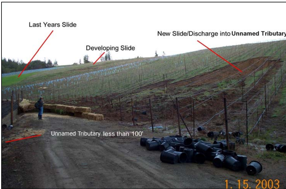
Figure 5. Landslide on south-facing slope of north unit; drainage to NF Mud Springs Creek in early 2003. The straw bales stacked two rows high along the wire mesh fence retained a majority of the coarse grained soil; however the surface drains and roadway funneled substantial sediment into the nearby salmon-bearing stream between sediment monitoring Stations C and D. A larger landslide occurred at approximately the same location during the previous winter; still evident by the different ground cover planting and lack of grape stakes. Silt deposits on tree trunks between the road and NF Mud Springs Creek record the evidence of 1-2 feet sediment burial. The landowner installed subsurface drainage in the slope and 3 sediment retention/settling basins between the road and stream in summer 2003. At least one of these basins ruptured during winter 2003-04 (see Figure 60).
