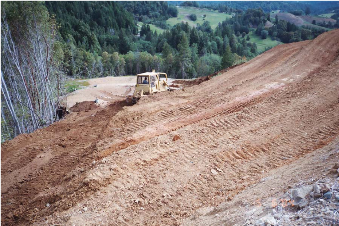
Figure 9. New terracing on south unit that drains into SF Mud Springs Creek, May 2004. Riparian stand on left is the upper end of the tributary stream that flows in between sensors at monitoring Station B. Terraces create steeper slopes over half the surface area. The dozer had pushed soil into the head of this steep head of the stream that is likely to experience high sediment concentrations next winter. New terracing was also completed above monitoring Station C in NF Mud Springs Creek during 2004.
