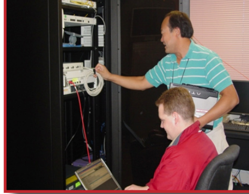
{ Carmody Rauch (seated), U.S. Army Information Systems Engineering Command wireless lead engineer and Rodney Hom , IT engineer, conduct Unified Capabilities Approved Product List (UCAPL) tests in the wireless lab at Fort Huachuca, Ariz. }
