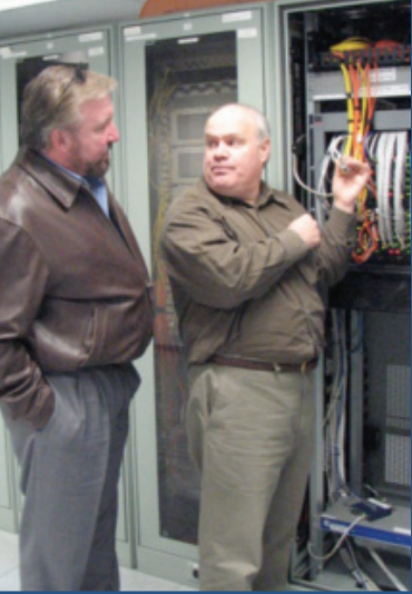
{ Bryan Kleese and Jeff Sleuter of USAISEC inspect fiber connections to an ATM switch at the Heidelberg Technical Control Facility. — Photo courtesy of USAISEC }
