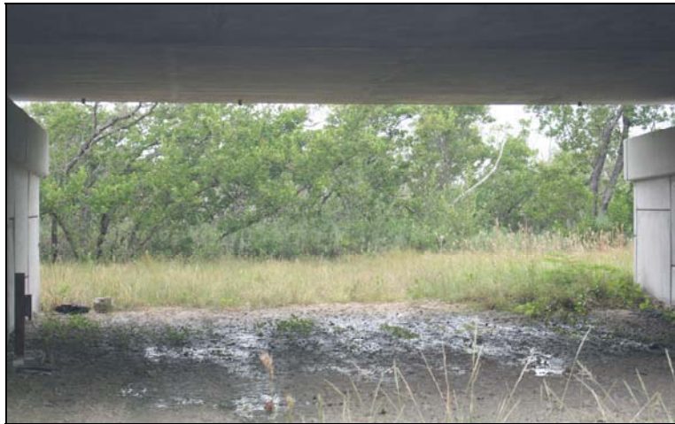
Figure 4.2: Example of a Key Deer Underpass
