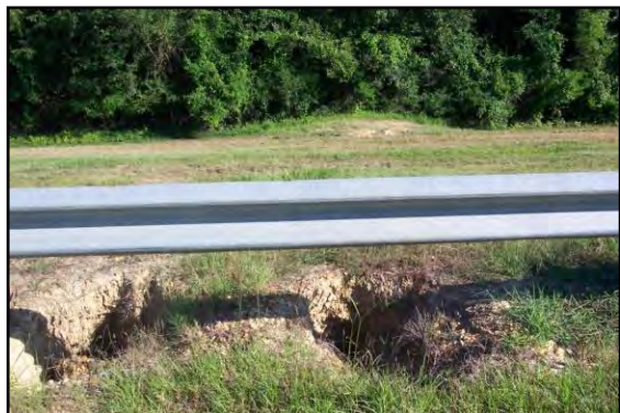
Photo Source: US Army Corps of Engineers Figure 2.6: Voids along Embankment (Typical)
