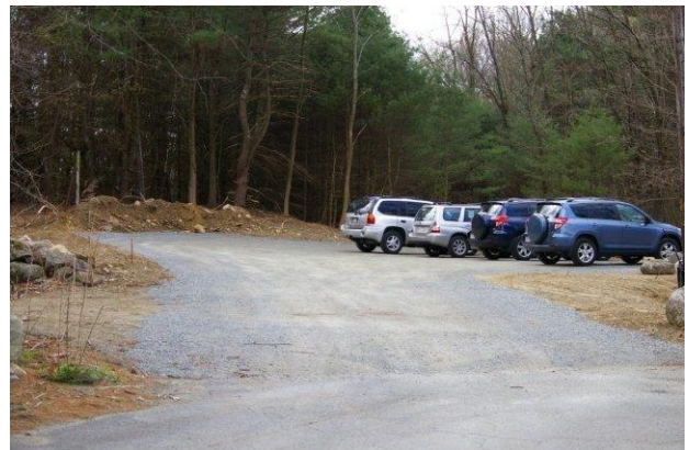
Visitors have begun to use the new gravel parking lot that is under construction at the East Entrance (Spring 2012).
