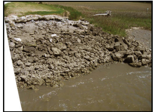
The northeast embankment is washing away.
