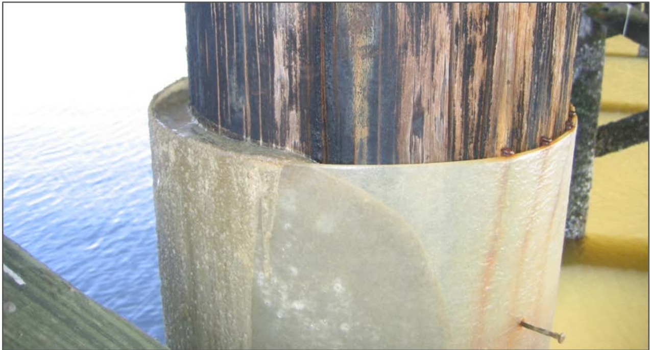
Figure 2. An existing FRP jacket is shown.
