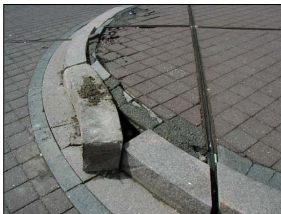
FIGURE 2-12: Misaligned granite curb
