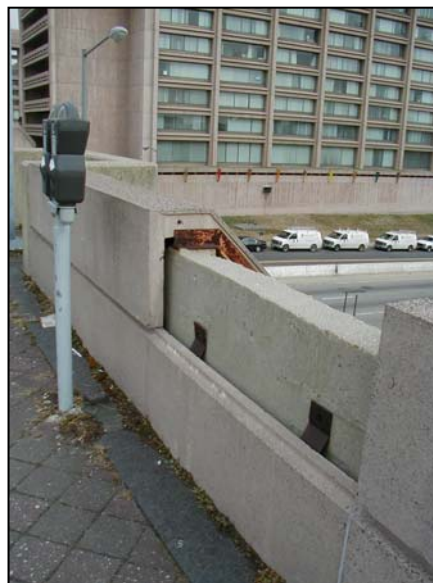
FIGURE 2-11: Missing canopy panel on I-395 bridge
