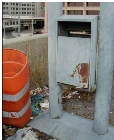
FIGURE 2-4: Deteriorating light standards and debris along Promenade
