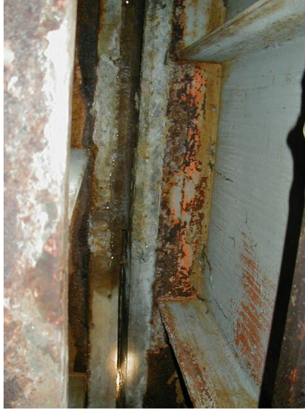
Photo 1: Active drops of water, and corroded top flanges of girders at deteriorated deck joint.
