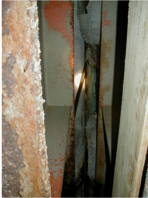
Photo 3: Attempted repair on slab and hanging joint filler material at deck joint.
