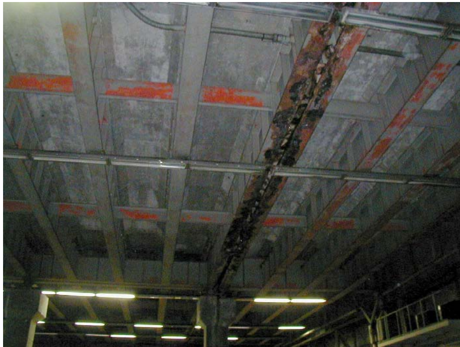
Photograph 7 Bridge No. 1114, showing deterioration of girders and beams.
