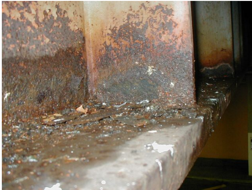
Photo 2: Moisture and corrosion found on top of bottom flange and lower areas of web and stiffeners on a girder near a failed joint.
