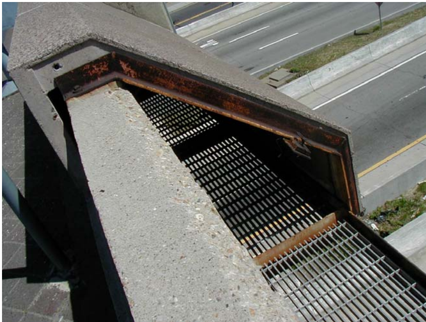
Photo 8: Steel frame used to help support precast panels; shown at location of missing panel on Bridge No. 1108.
