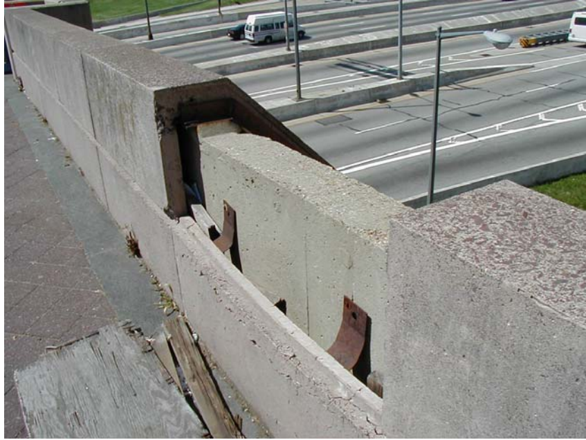
Photo 7: Missing precast concrete panel at parapet wall on Bridge No. 1108, over I-395/Southwest Freeway.
