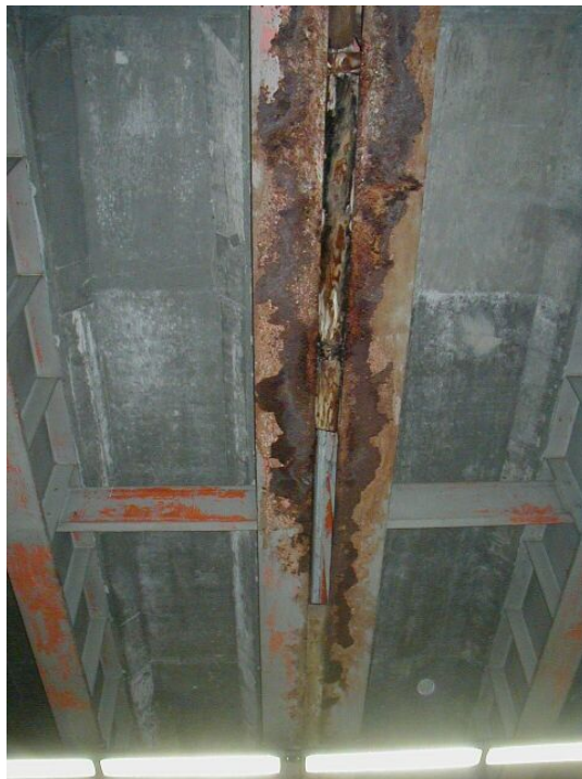
Photo 4: Typical corrosion found on bottom flanges of girders, and wood shoring located between them, at a failed deck joint.
