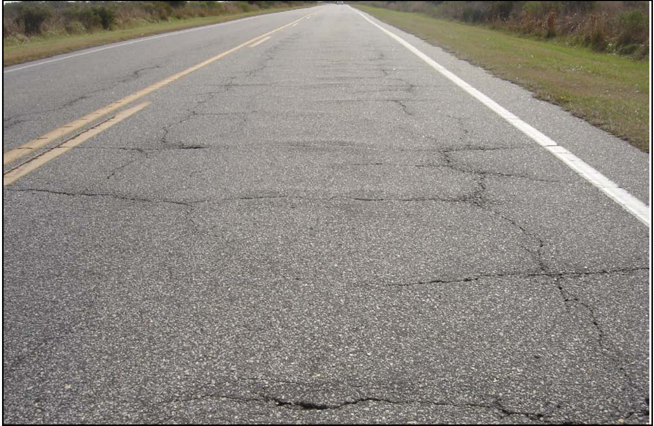
Figure 1. Fatigue cracking is apparent in the southbound lane of NC 12
