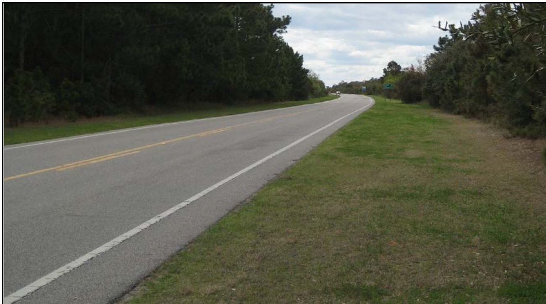
Figure 3. The existing stretch of NC 12 running through Cape Hatteras National Seashore has two-foot paved shoulders.
