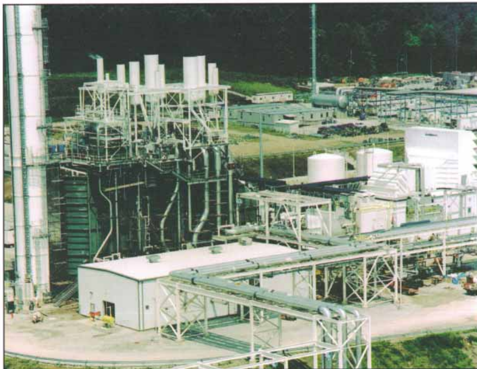
Wabash River gasifier/combustion turbine/HRSG train during construction. The pipe rack, foreground, connects to the repowered steam turbine Unit 1.
