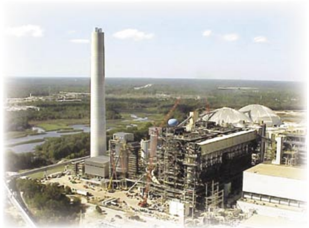
JEA plant with CFB boilers in center and fuel storage domes in background
