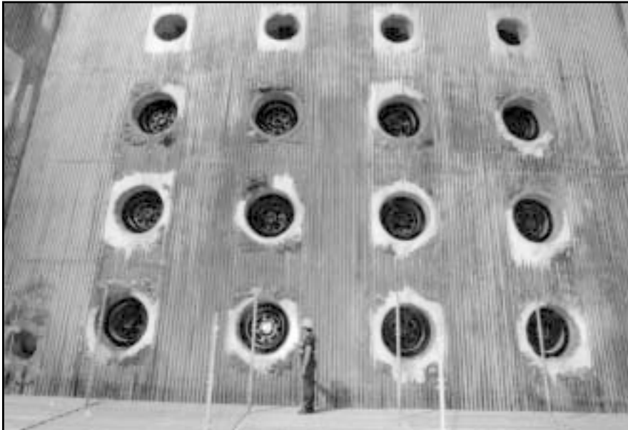
West wall of boiler with LNBs and AOFA installed
