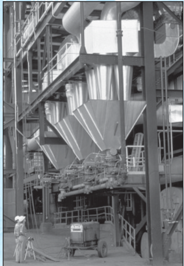
Plant Crist cyclones for SCR reactors.
