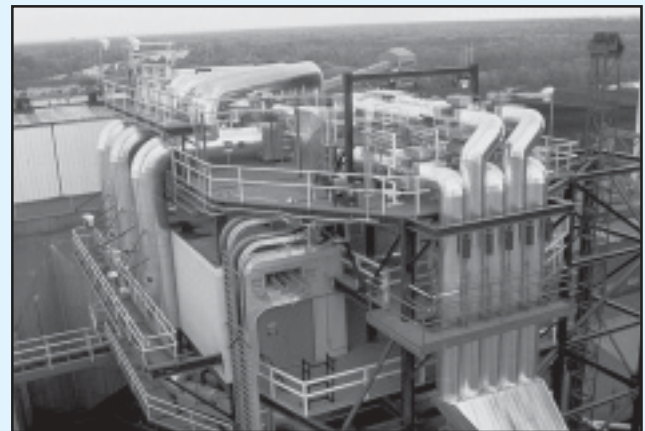
SCR test facility installed at Gulf Power's Plant Crist, Unit No. 5, a 75-MWe tangentially fired, dry bottom boiler
