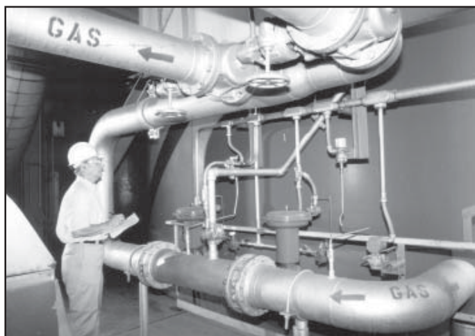
In-plant natural gas distribution lines for gas reburning
