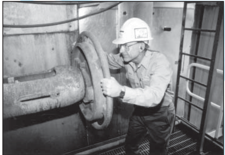
Main natural gas shut-off valve for the plant
