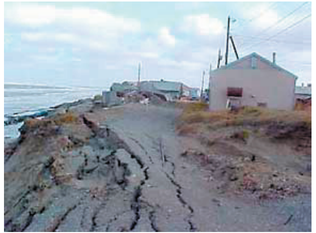
Facing massive coastal erosion, the Native Village of Shishmaref, on the Chukchi Sea in Alaska voted to relocate the entire community inland away from danger. (Courtesy of Tony Weyiouanna, Sr.)
