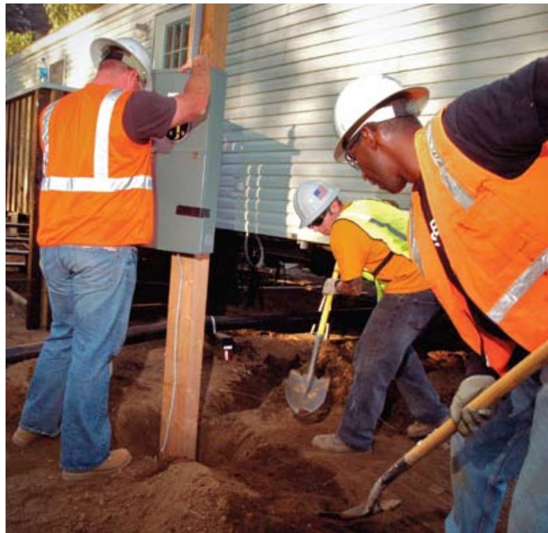
Delzura, California, December 5, 2007 – The electricians are connecting electricity to serve a family that will temporarily live in the FEMA – provided mobile home while they begin to rebuild. The family lost their home during the wildfires in October.
