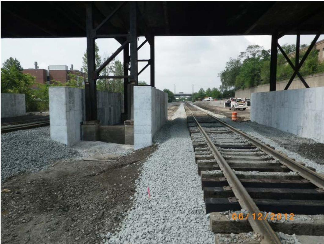
University of Akron Overhead Walkway (OH) after removal of platform and lowering of tracks
