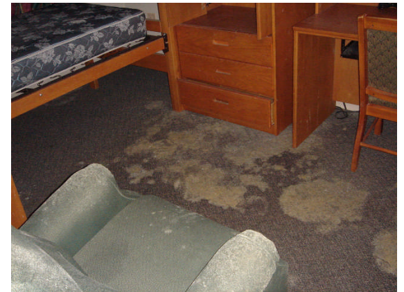
Barracks Room, Humidity >60%
