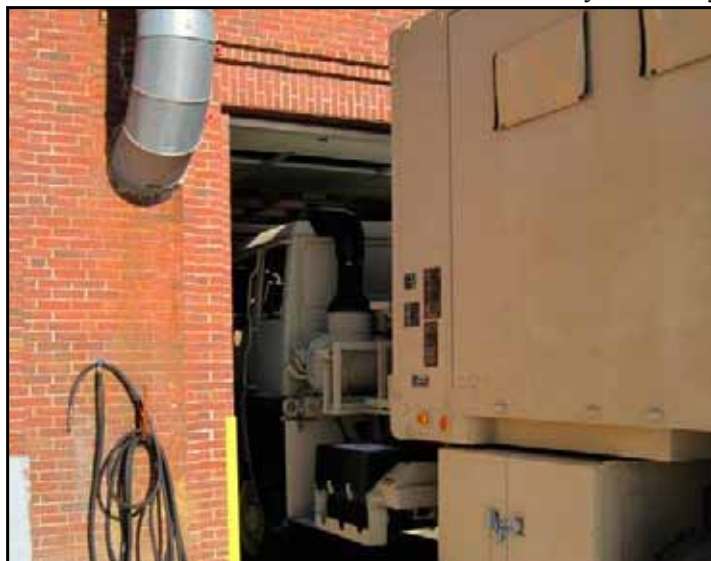
Note that the LMTV Truck will not fit into the bay door fully.
