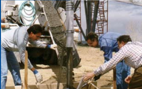
Duane Whitcomb, Ken Eis and Michael Hiatt putting in the antenna base for the GOES data collection.
