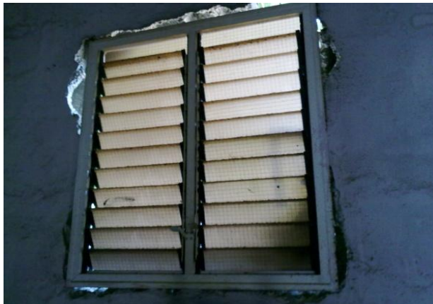
Installed window has large gaps between the window frame and wall. (Photo by audit firm contracted by RIG/Cairo)
