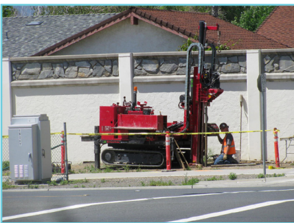
A drilling specialist positions a track-mounted drill rig to install a test boring. Soil samples from the boring were inspected to characterize subsurface soil conditions.
