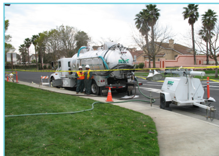
Two field technicians monitor the performance of a vacuum truck as it removes jet fuel from a soil boring near the fuel leak.
