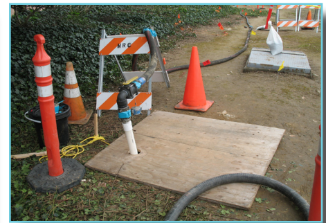
A suction tube that is connected to a vacuum truck removes jet fuel in the ground after it was released from a leaking valve.
