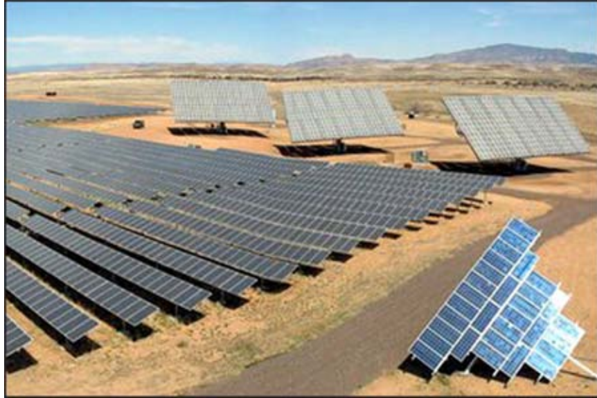
1 2 FIGURE F.3.2-1 A Utility-Scale Flat-Plate PV System at the 3 Prescott, Arizona, Airport Operated by Arizona Public Service 4 Company (This system incorporates flat-plate nonconcentrating 5 solar panels [foreground] and concentrating flat-plate solar 6 panels [background].) (Credit: Arizona Public Services; 7 Source: NREL 2010) 8 9
