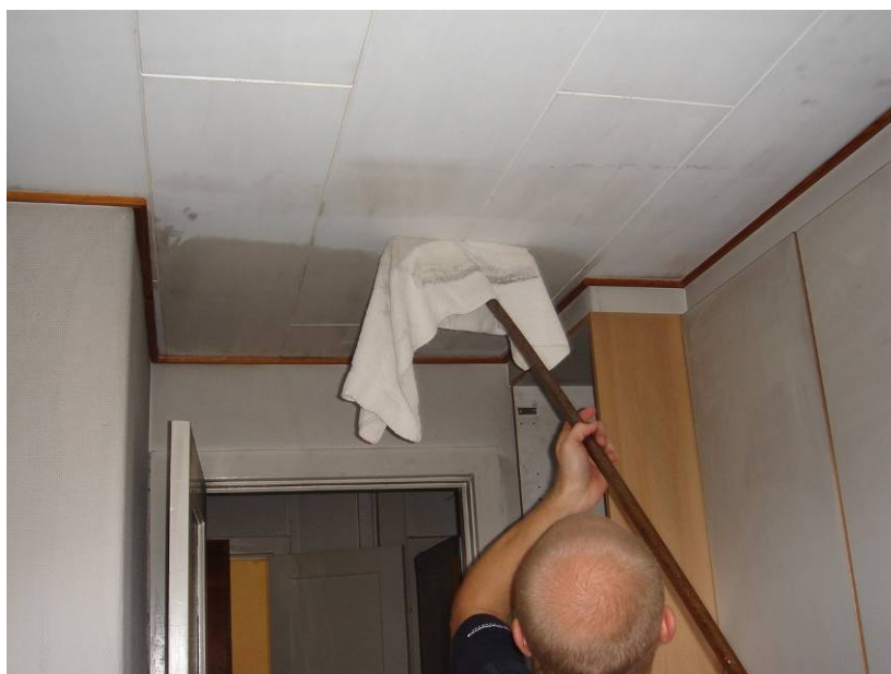
Photo 2: Cleaning of ceiling in soot-damaged flat.
