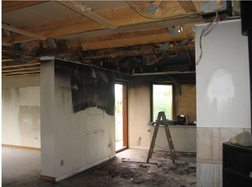
Photo 4: The fire started in the living room and burnt the ceiling. The carpenters have just repaired the damaged rafters.
