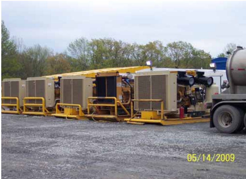
Photo 6.1- Electric Generators, Active Drilling Site: Source: NTC Consulting
