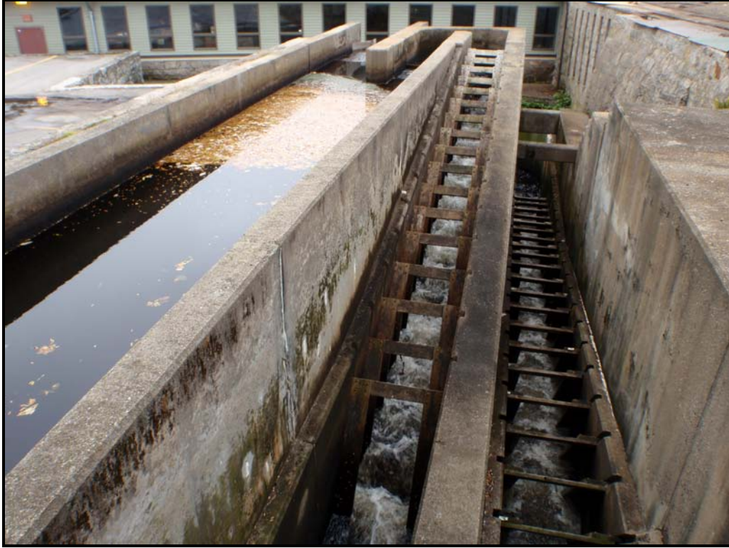
Figure 4. Palisades flume (left), fishway (right), and proposed work site of the central wall extension, looking from upstream of the structures, 2011, Saugatucket River, Peace Dale, RI
