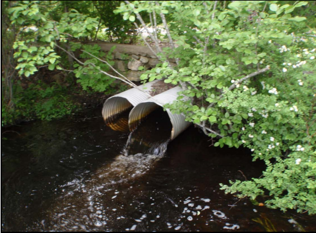
Figure 6. Teal Drive culverts, Factory Brook, South Kingstown, RI, 2011. The culvert perched on the right is higher than the culvert on the left and both culverts provide poor fish passage with varying stream flows.
