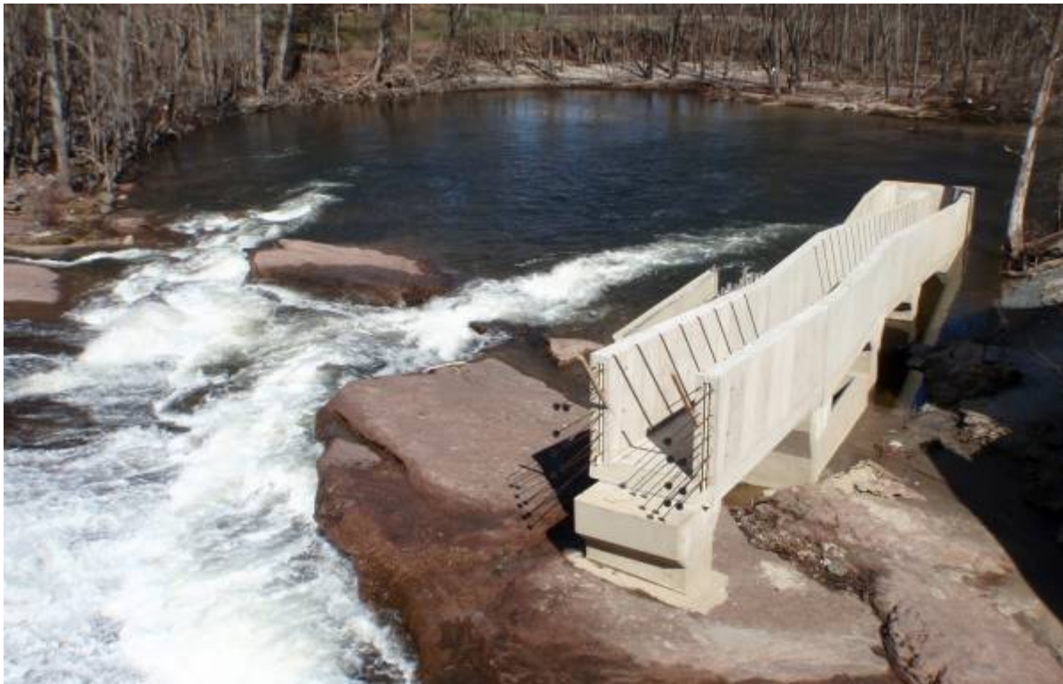
Figure 6. Partially completed Manhan River dam fishway in Easthampton, MA. Settlement funds would contribute to the overall funds needed to complete the Denil fishway for anadromous fish passage.
