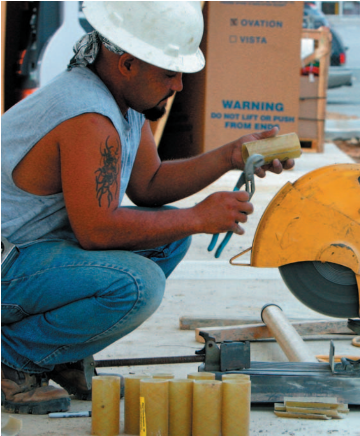
Construction accounts for nearly 5 percent of the U.S. economy; here a worker fits pipe on a gasoline station under construction in Georgia.
