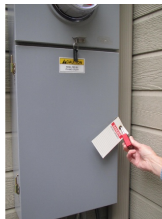
Figure 15. Lock out the electricity panel and verify that the circuit is de-energized
