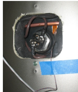
Figure 20. Surface-mounted TC at the lower tank surface
