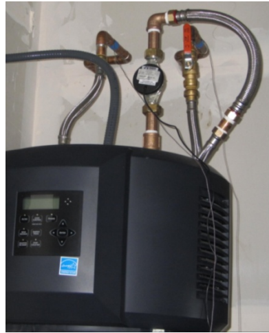
Figure 17. Final plumbing configuration with the flow meter and an extra length of flexible pipe installed
