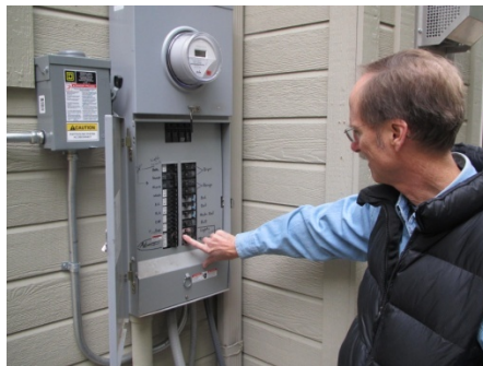
Figure 14. Turn off the breaker for the HPWH.
