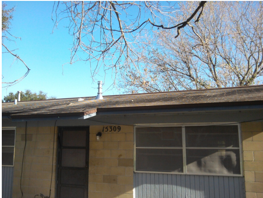
Figure L.2. Actual vertical venting assembly attached to the roof
