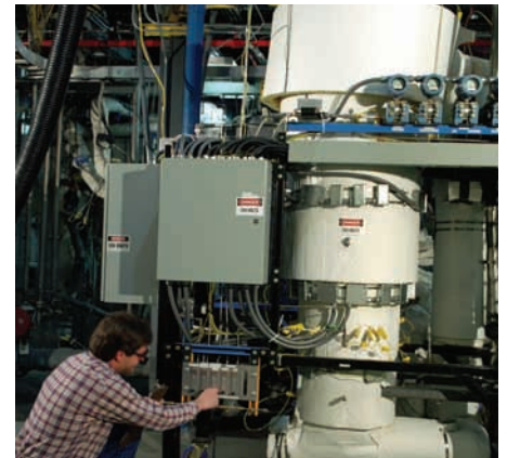
Novel technologies to increase the efficiency and lower the cost of biomass conversion are validated at the pilot scale. Photo: NREL/09706
