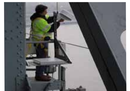
An employee from the Center for Operational Oceanographic Products and Services installs an air gap sensor which measures bridge clearance on the Verrazano-Narrows Bridge, New York. The sensor is part of the New York/New Jersey Physical Oceanographic Real-Time System. Information from the sensor is critical for under-bridge clearance, as ships continue to maximize channel depths and widths while, at the same time, push the bounds of bridge heights
