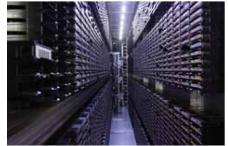
Massive tape library transitioning to new Enterprise Archive System
