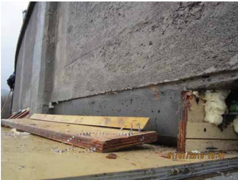
Above: A small portion of the new deck is revealed. The outside visible face of the new deck will be sandblasted once all concreting is complete.
