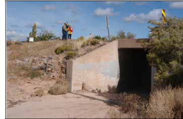
Arroyo embankment and culvert headwall adjacent to NM4 in the residential area. The RSA Team members are standing on the narrow shoulder adjacent to this embankment and headwall.
