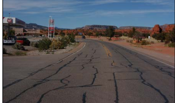
Looking north along NM4 at the Red Rocks recreational area. Roadside land uses include the commercial area (service station and Walatowa Visitors Center) visible at left, and the recreational area (where small-scale vending takes place during the summer) at right. The speed limit along this segment of the highway is 50 mph.
