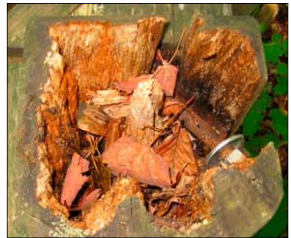
Figure 9. Examples of internal decay in vertical members that were cut to height after installation. Only the preservative-treated zone remains sound. In some sawn members with heartwood faces, the shell may not be complete (see photograph on bottom). Fortunately, most pressure-treated members used in bridges have greater penetration than shown in these examples.
