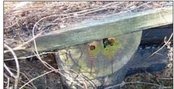
Figure 11. The older pile pictured on the bottom demonstrates how decay eventually develops in the untreated core of piles that have been cut to height on the job site. Cutting the piles at an angle with the intent of encouraging water to run off does not inhibit decay.
