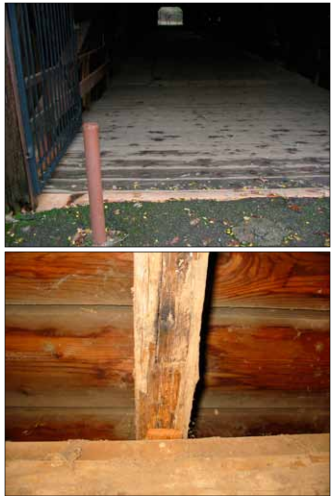
Figure 4. Members at ends of covered bridge are vulnerable to wetting from wind-blown rain. The picture at the bottom shows decay in a stringer under the bridge decking shown on the top.
