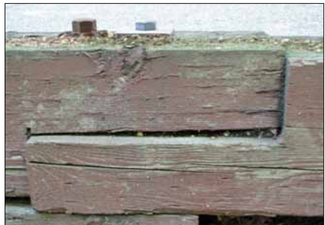
Figure 16. Unless it was pressure-treated after fabrication, this type of connection is a recipe for decay. It exposes untreated wood and creates an area that traps and holds moisture.
