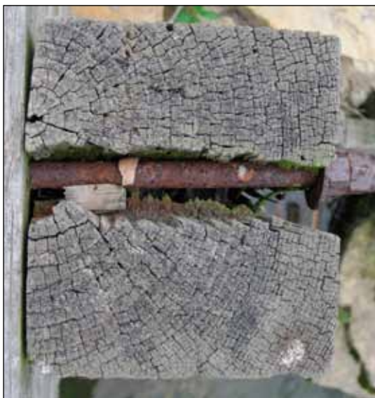
Figure 14. Metal fasteners are sometimes associated with decay pockets if holes are drilled after treatment and expose untreated wood. Field-fabricated bolt holes should be field treated with a preservative such as copper naphthenate during construction.
