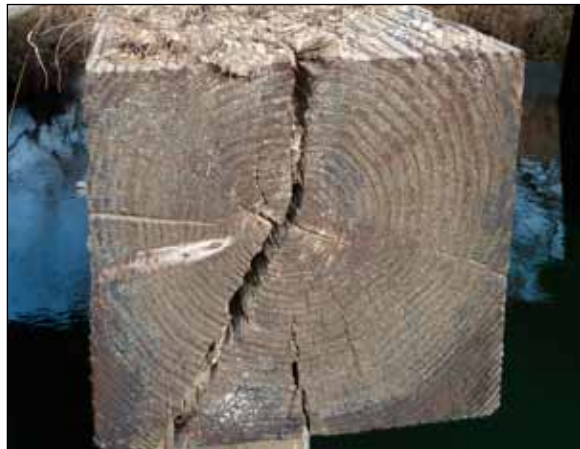
Figure 13. Checks allow ready access for moisture from rain and snow to reach the interior of large timbers. An accumulation of organic matter further increases the potential for decay.
