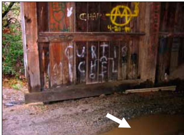
Figure 18. Puddles near bridge entrances cause lower members to be repeatedly wetted by splash from vehicle traffic.
