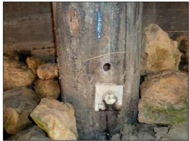
Figure 15. The upper bolt in this pile was either removed or never installed. The hole now serves as a ready access for fungi to the untreated interior of the pile.
