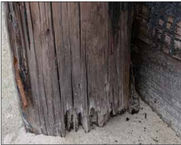
Figure 17. The groundline area of piles represents a severe decay hazard.
