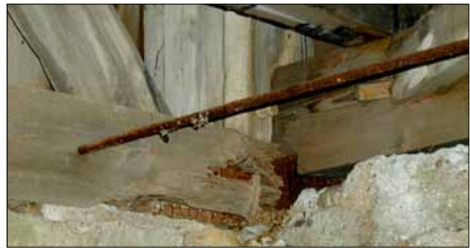
Figure 3. The area where covered bridge members contact the abutment or supports at the ends of the bridge often provides conditions for deterioration.
