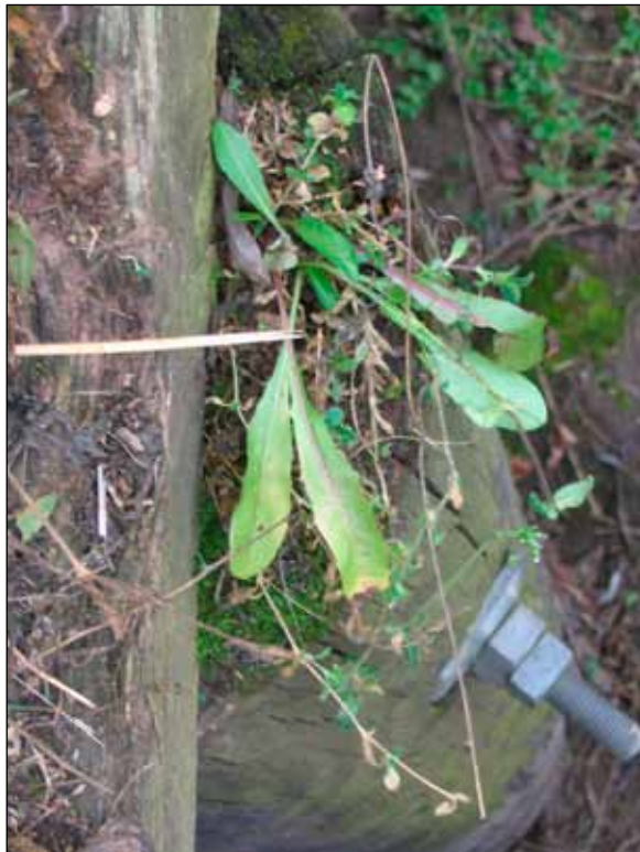
Figure 10. These piles are at risk of developing internal decay, and it is likely that the pile on the bottom already has substantial decay. Although cutting piles to height after installation is a common practice, the exposed untreated wood should be field treated and then protected with a durable cap. In this case, the tops are only partly protected, and organic matter is accumulating on the pile tops.
