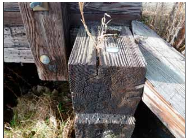
Figure 19. Vegetation growing on a structure is an indication that conditions are favorable for decay.
