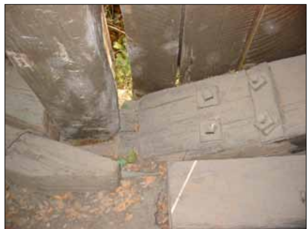
Figure 20. This type of accumulation of dirt and organic matter makes decay more likely and more rapid if moisture reaches this area.
