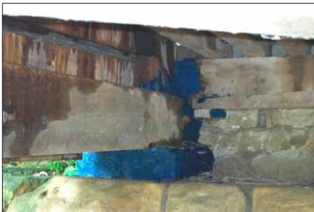
Figure 41. Example of application of a copper-borate paste to the members contacting a bridge abutment.
