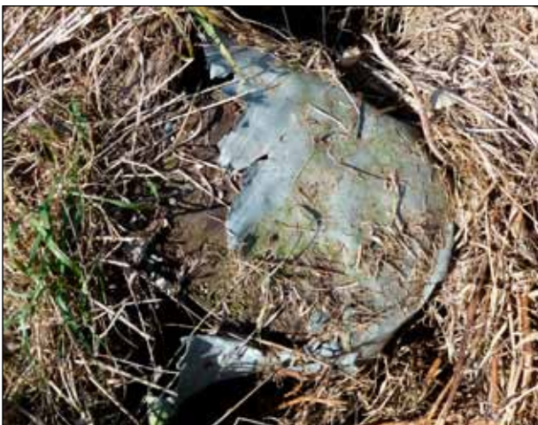
Figure 22. Galvanized pile caps (top) can provide protection of cut surfaces if applied at the time of construction. However, pile caps alone do not stop decay that has already started, and they must be inspected to ensure that they have not been damaged (bottom).
