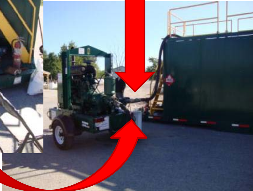
Self-powered Circulating Pump
