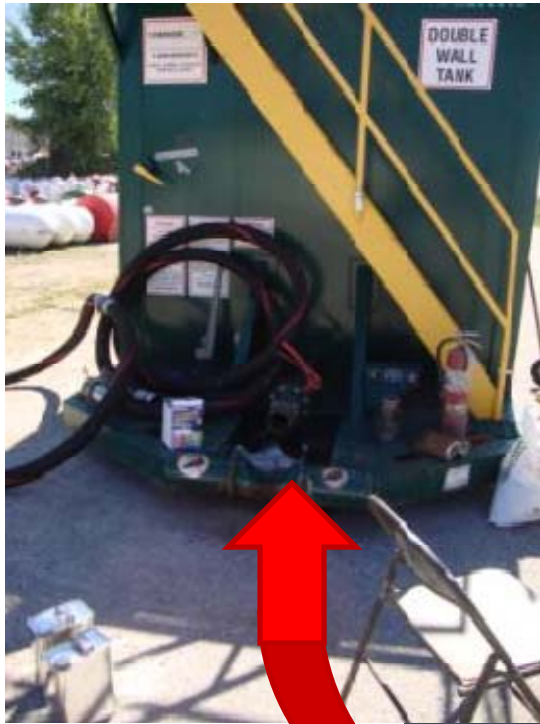
Suction from front, bottom of tank
