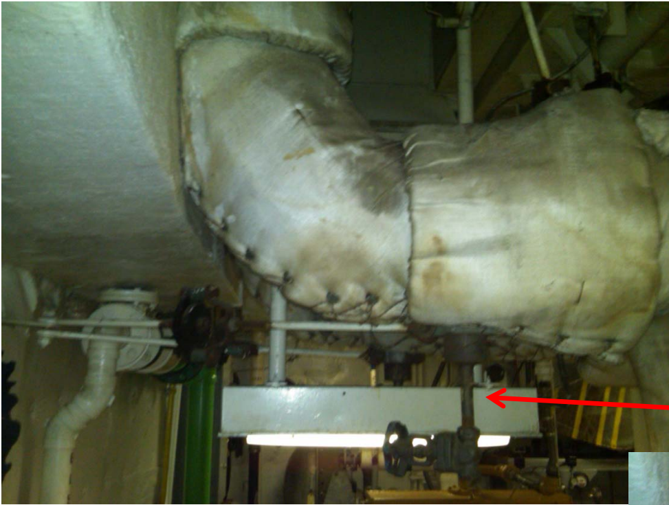
DG #4 Exhaust Trunk with blanket
