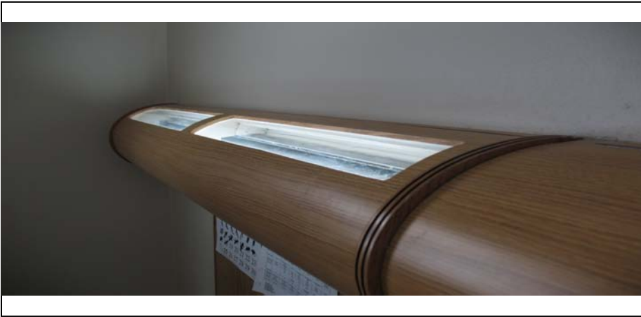
Figure 3.2.5.10: Over-bed Light Fixture
