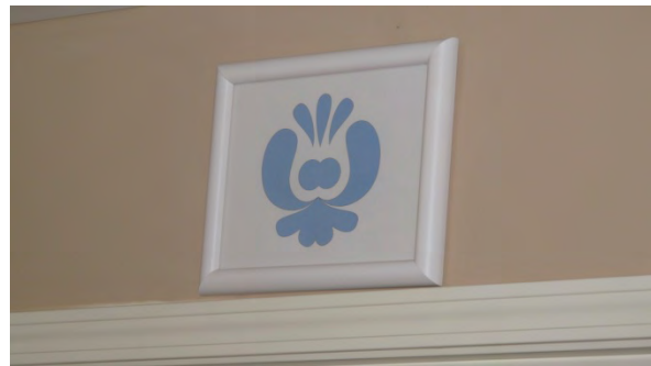
Figure 3-63 Above Resident Room Door - Artistic Emergency/Nurse Call Light Lebanon Valley Brethren Homes
