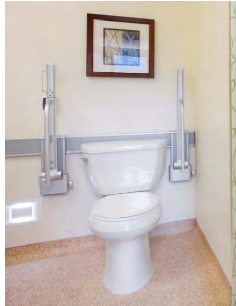
Figure 3-15 Fold-up Grab Bars in Toilet Room NewBridge on the Charles
