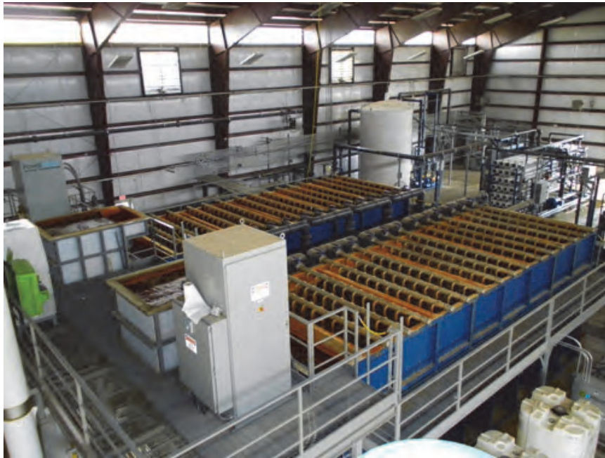
Figure 25. EC and RO treatment system (Courtesy of Scott Powell, 2012).
