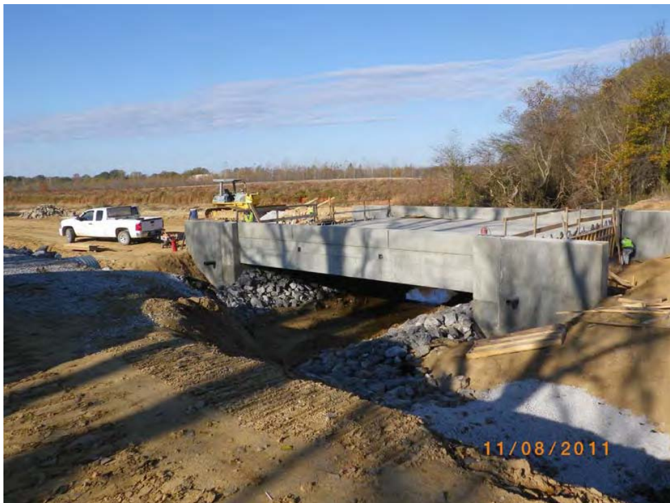
Construction of the "Y" Bridge near the main tracks at the Memphis Intermodal Facility
