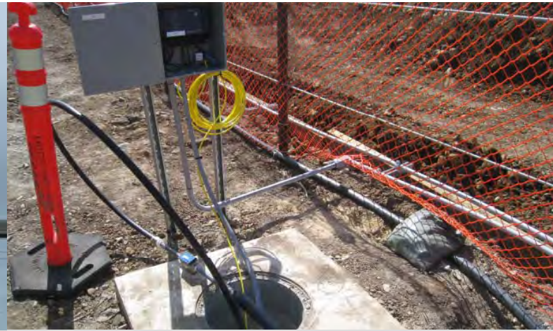
DW-04 – Dewatering Well
