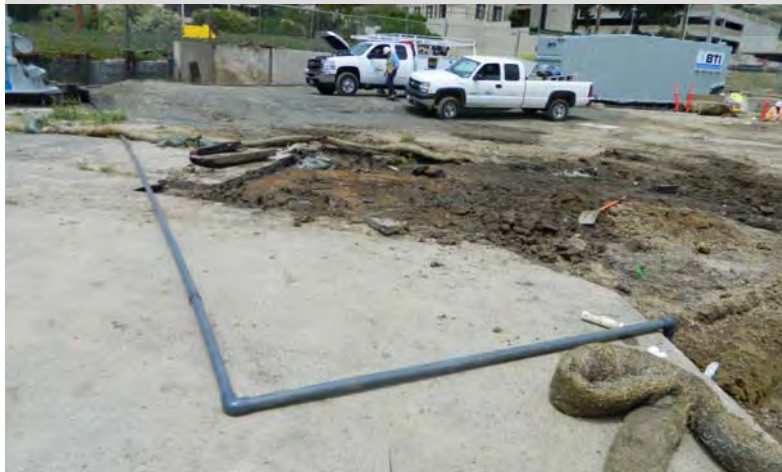
Temporary Water Line
