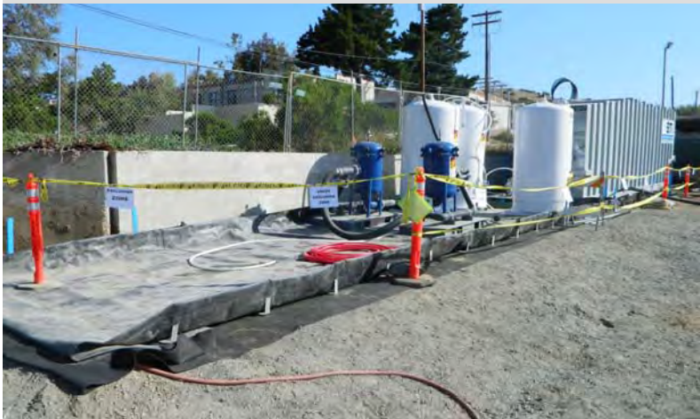
Treatment System – Bag Filters and Granular Activated Carbon
