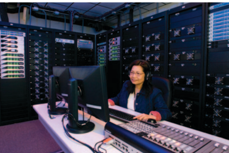
Phuong Tran configures an experiment in the Control Room. Rack-mounted equipment is used to control the stimulus presentations in the research space.
