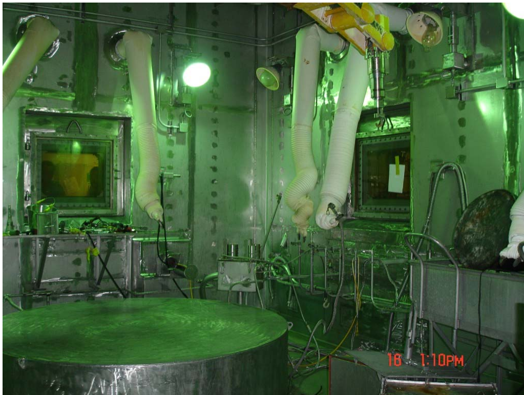
Figure 10. New Waste Calcining Facility Cell 308 interior.
