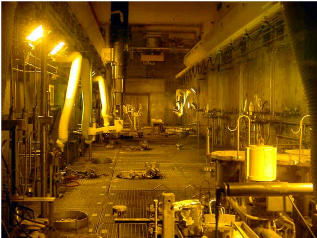
Figure 11. Current view of Fluorinel Dissolution Process cell at 0-ft level (looking south).
