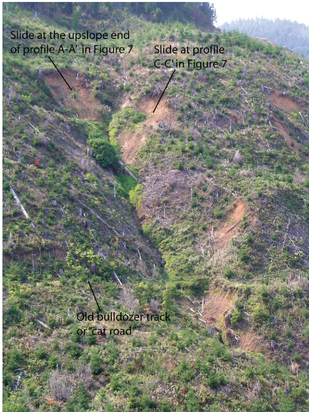
Figure 11. Photo of site 3s5w30-11. Plan and profile data of the site are shown in Figure 7.
